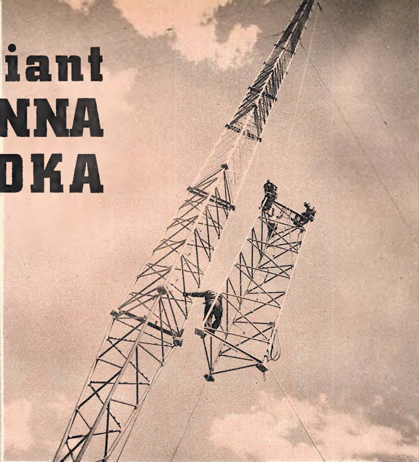
KDKA's new 718-foot antenna is composed of 32 three-cornered welded steel sections placed one atop another (above). The 60-ton structure rests in a ball-and-socket joint of a huge porcelain insulator, as shown at left.
